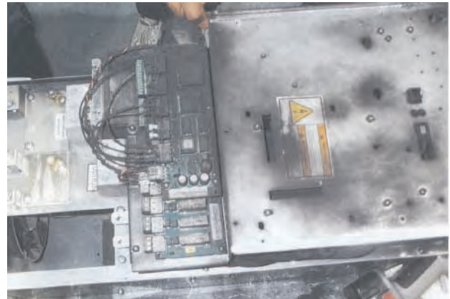
Photo 1, Fan Injecting Dust into Drive Enclosure
