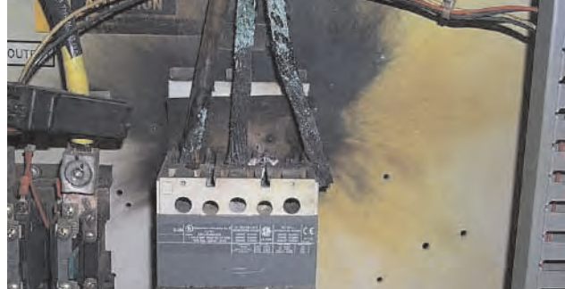
Photo 3, Arcing Caused by Loose Input Contacts
